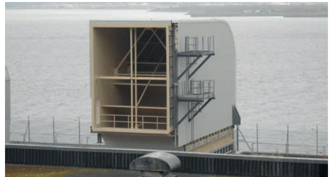
Clean Gas Duct lined with COROFLAKE 24
