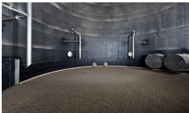
Floor of an absorber rubber lined with CHEMOLINE 4 B and additional brick lining with CHEMOKITT FU 1310
