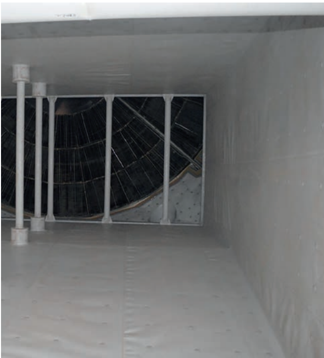
PTFE-M lining in a raw gas duct
