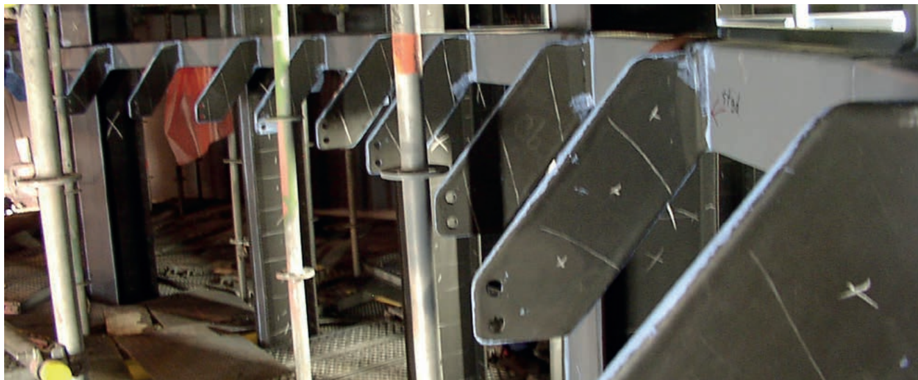
Rubber lined supports in an absorber
