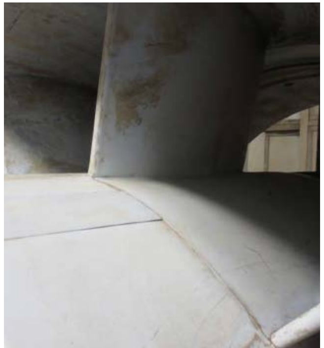
REMAFLON (PTFE) as nonstick lining in a flue gas fan
