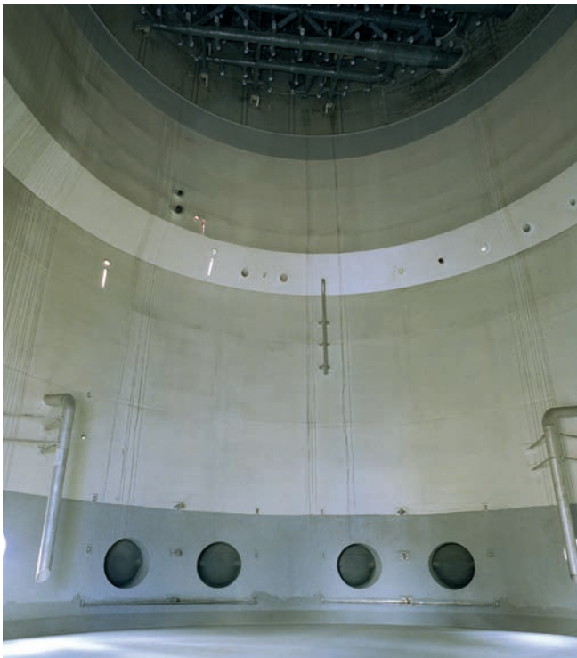
Lined flue gas scrubber
