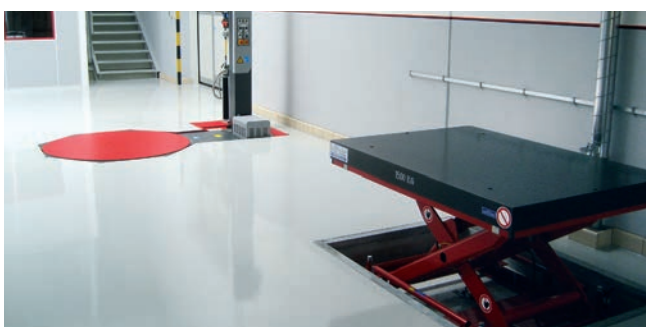
Conductive WHG coating in a production hall
