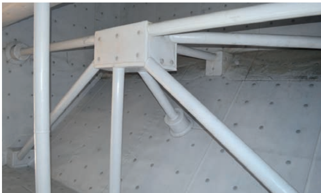
PFA lining in a raw gas duct
