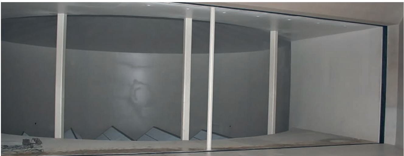
Coated clean gas duct
