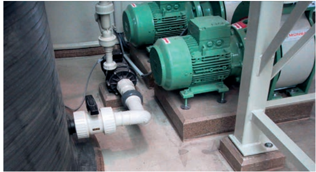
Polly-concrete bricks as pumping equipment foundation
