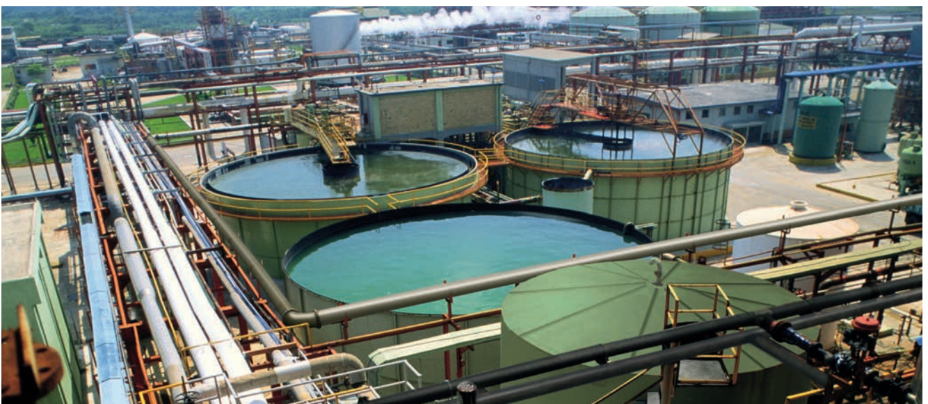
Rubber-lined sedimentation tank
