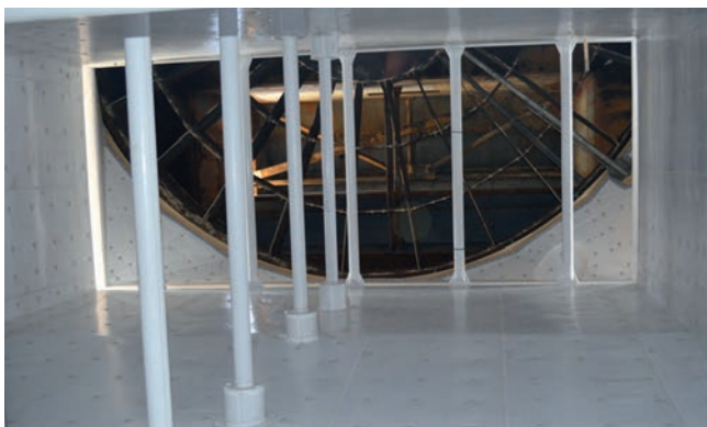
PFA lining in a raw gas duct
